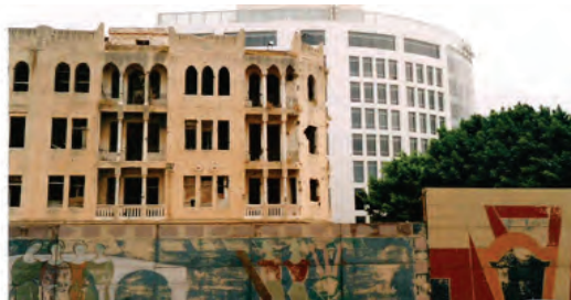
Figure 10. Beirut architecture damaged after the Lebanese Civil War (Source: Tarek Adelsalam)
