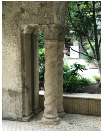
Figure 7. Spiral columns in the porte-cochere with their bases restored; notice how the ground level was lowered to achieve this. Photo by author.
